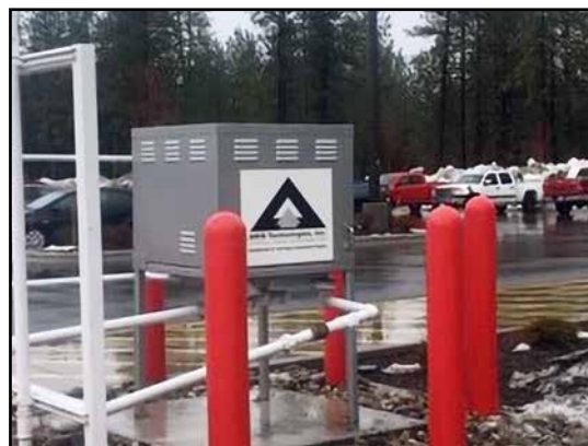
Pictured above is the permeator which collects the gasoline vapors from the vapor recovery systems.
